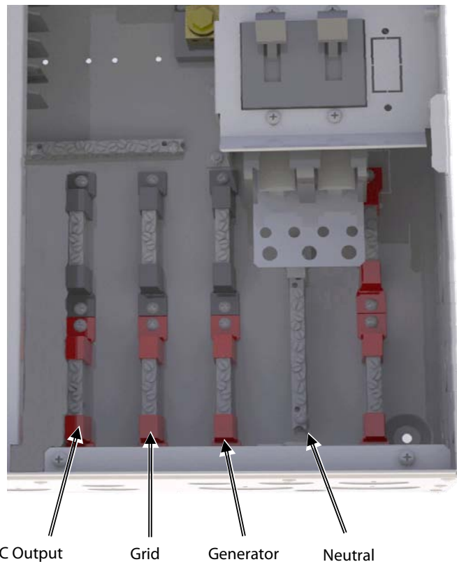
Figure 28 AC Terminal Bus Bars
