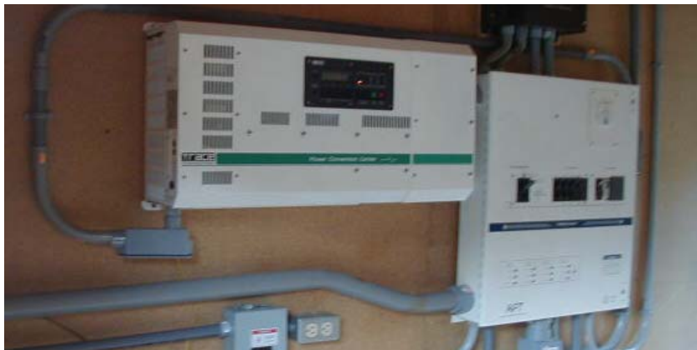
Ananda Power Center with a Trace SW and conduit box
