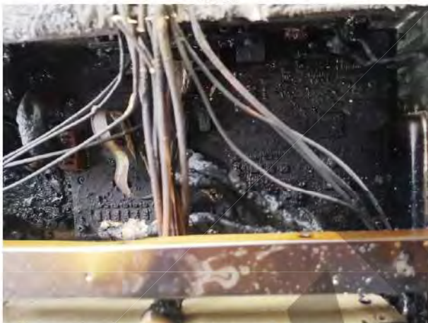
Figure 21c. Photo 02 of thermal runaway location.
