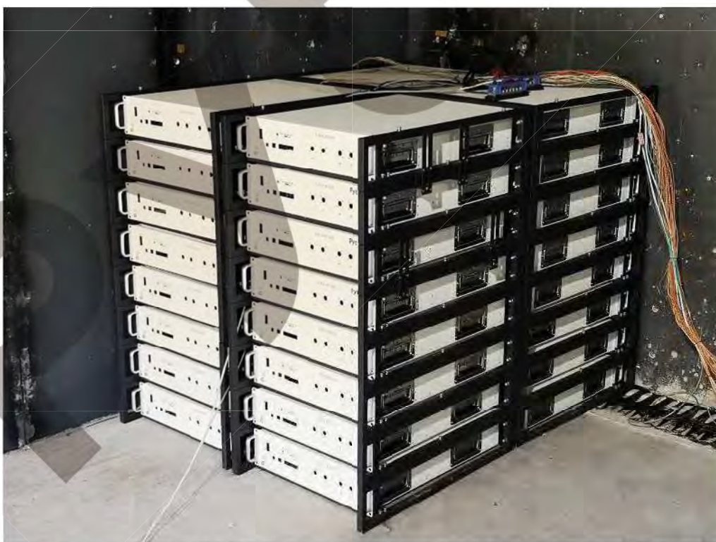
Figure 16. Photo 02 of initiating BESS unit and target BESS units after test.
