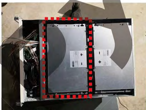
Figure 5c. Internal view 03 of battery module.
