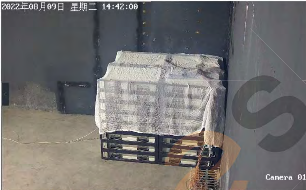
Figure 12. Photo 01 of initiating BESS unit and target BESS units during test.
