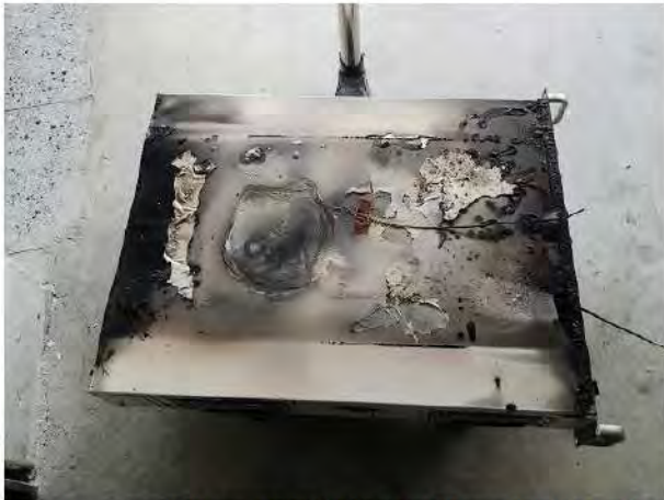
Figure 21a. Photo of initiating battery module after test.
