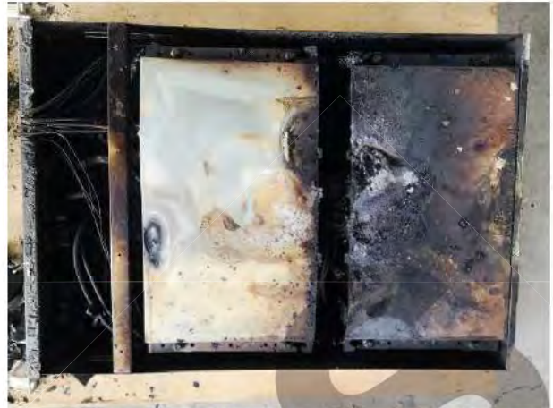
Figure 21b. Photo 01 of thermal runaway location.
