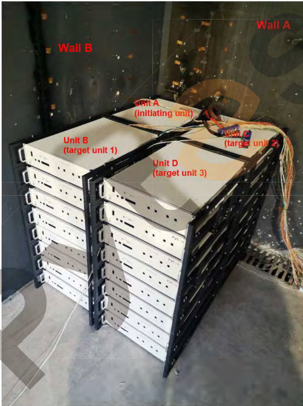
Figure 7. View of BESS within test room.
