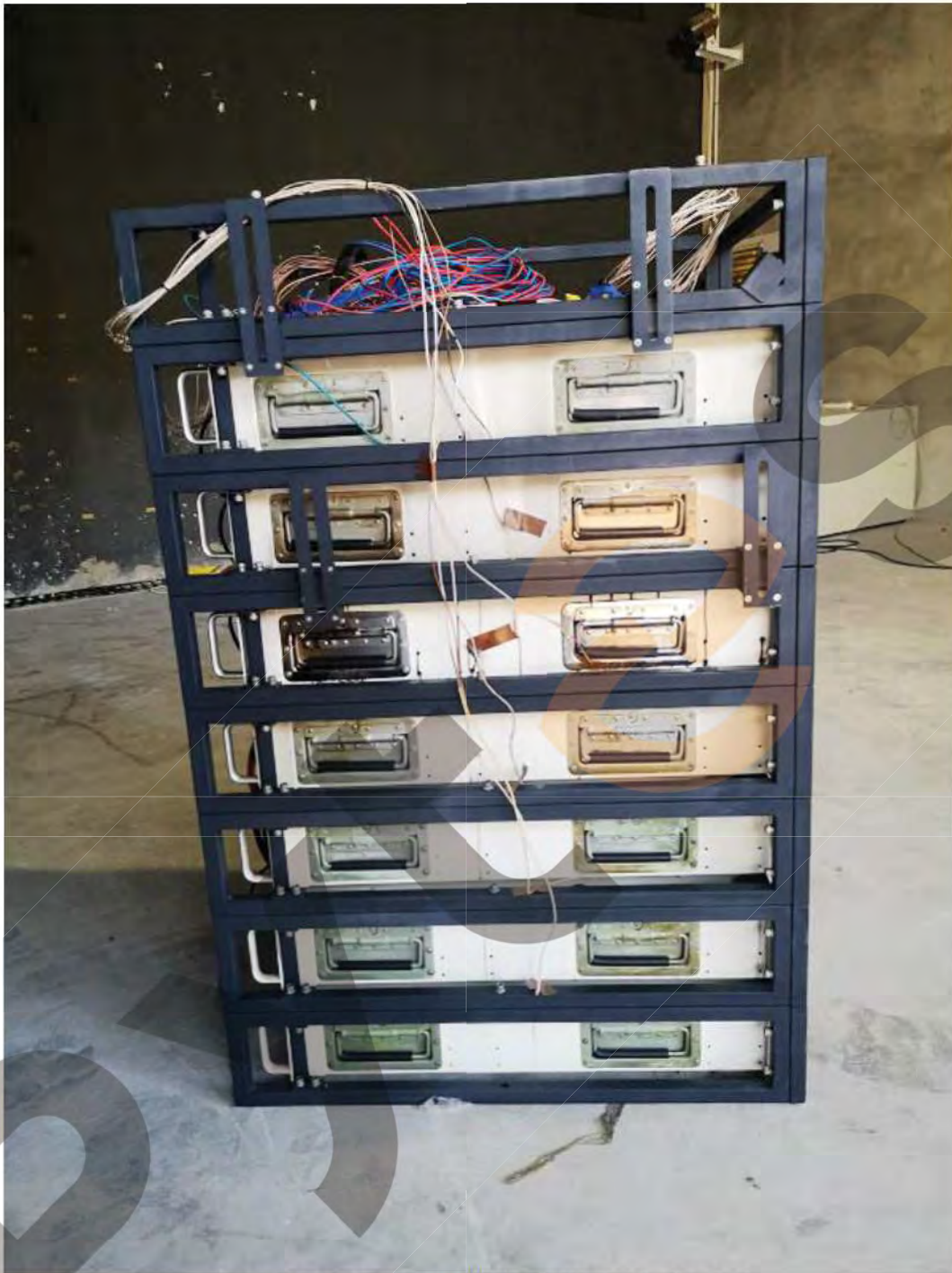
Figure 20. Photo 02 of initiating BESS unit after test.
