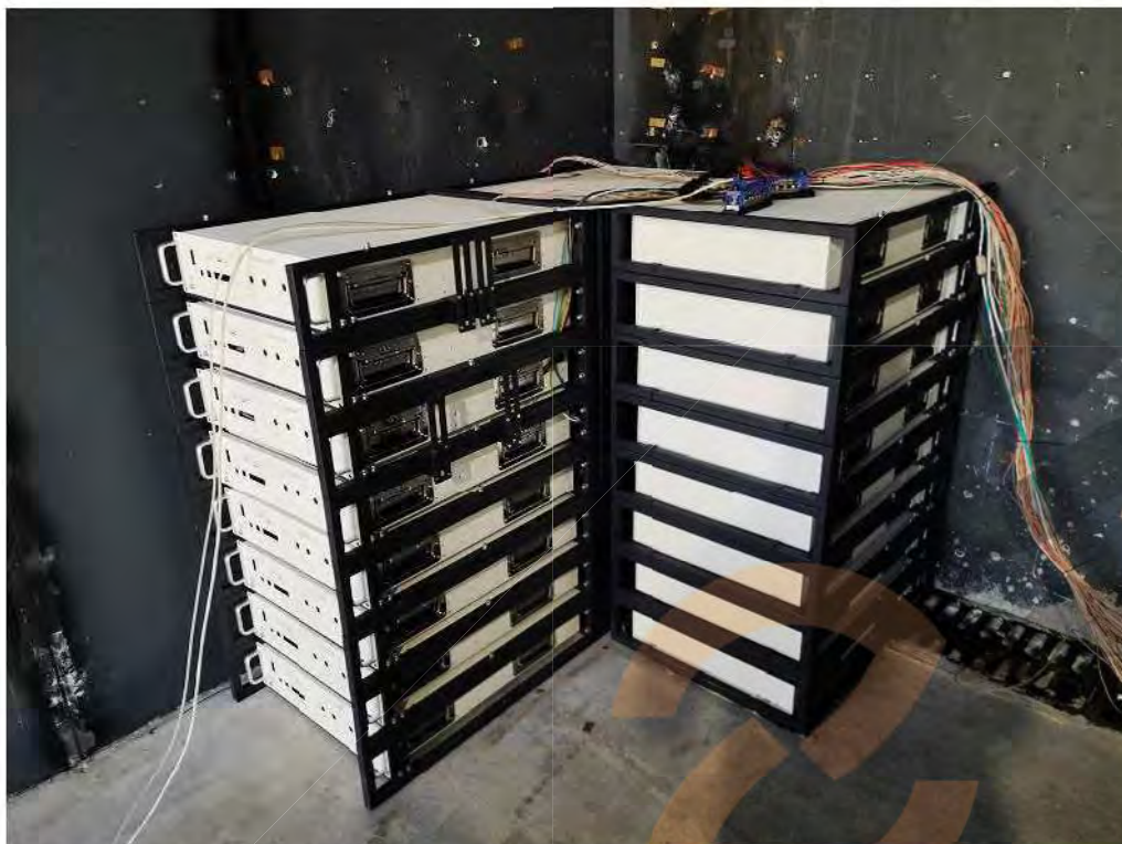
Figure 17. Photo 03 of initiating BESS unit and target BESS units after test.
