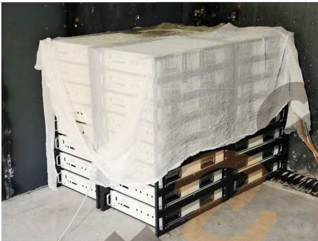
Figure 15. Photo 01 of initiating BESS unit and target BESS units after test.
