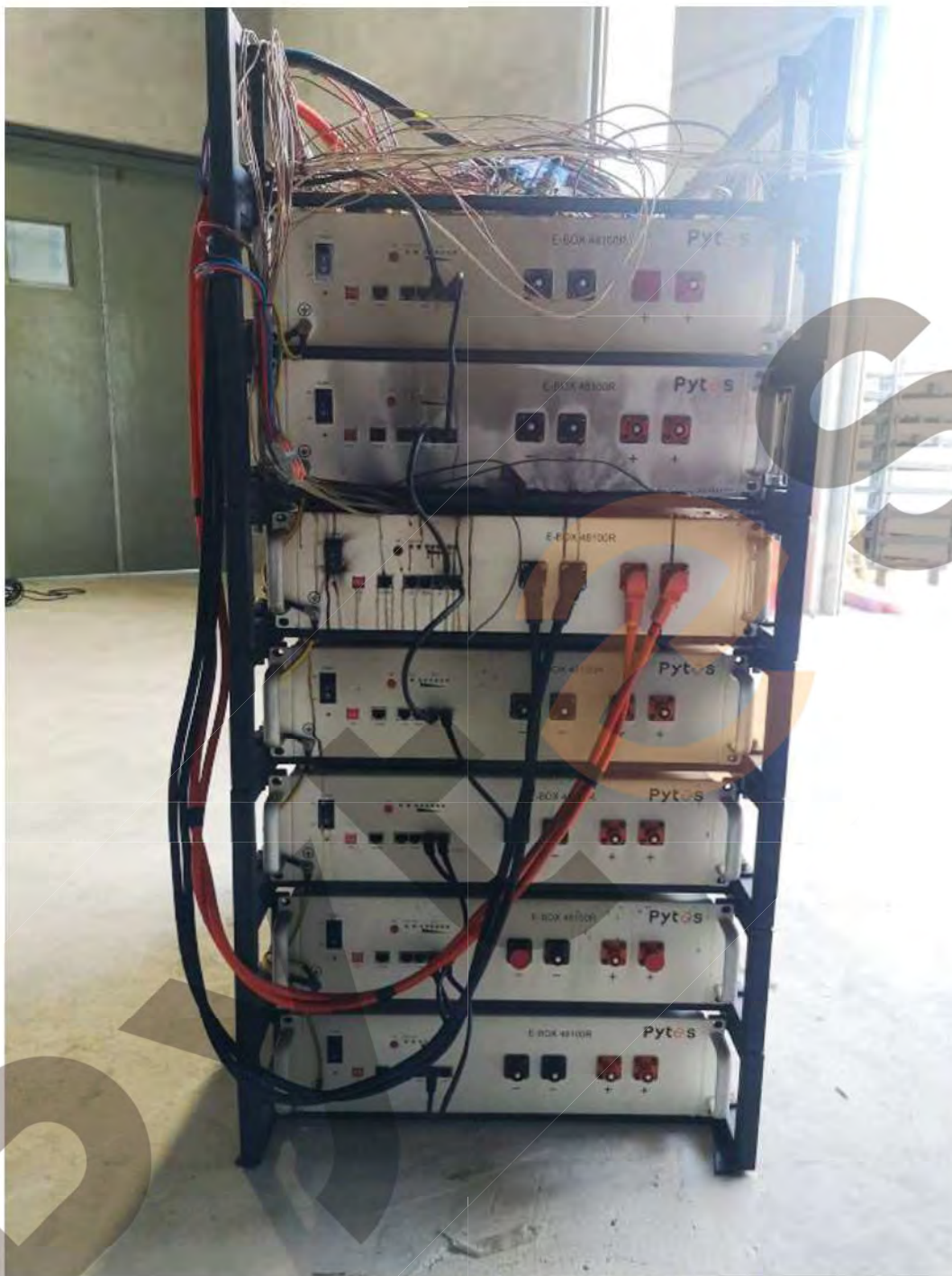
Figure 19. Photo 01 of initiating BESS unit after test.
