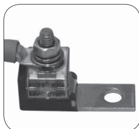
Fig. 3.9. Fuse MRBF and Positive cable fixed to the CFBAR
